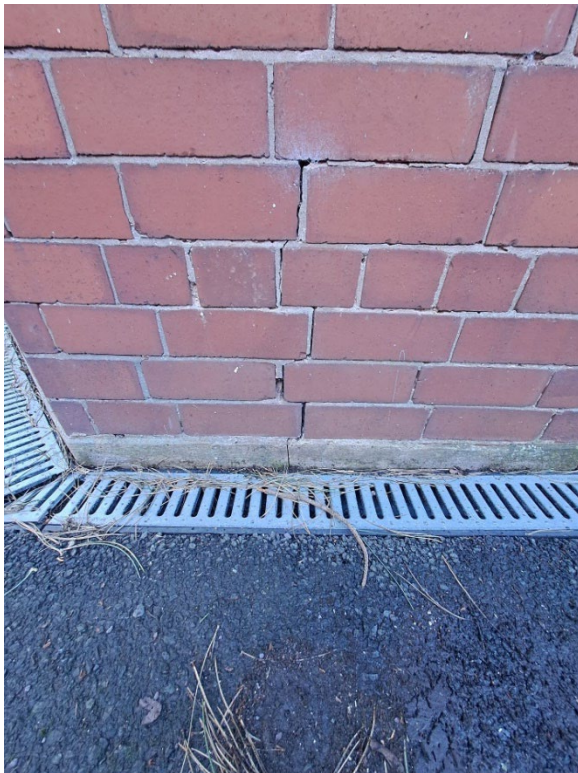
Image 1: Cracking in exterior wall
